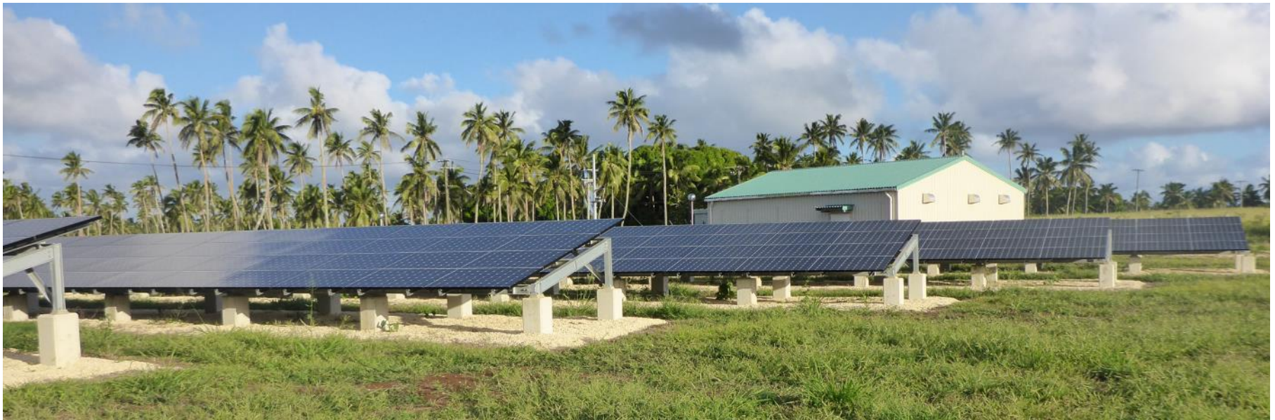
Tonga, Vaini Solar PV and Lithium Ion Battery Building
